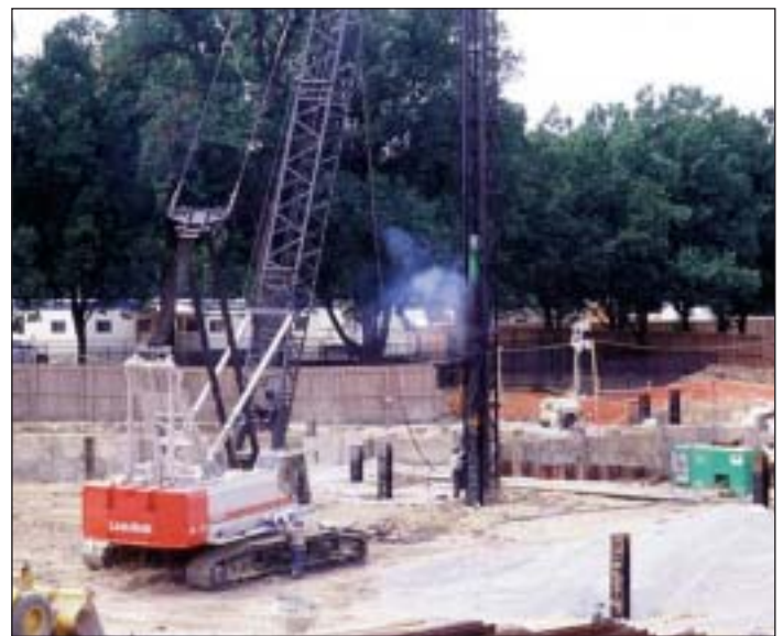
A crane drives a steel pile into bedrock. Nearly 600 steel piles will support the memorial’s concrete foundation. (Photo by Richard Latoff)
