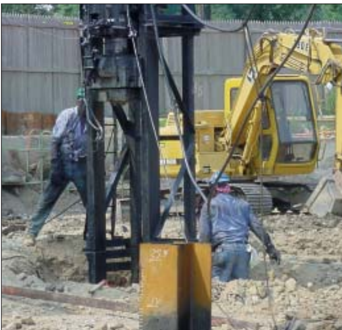
Workers monitor the progress of a pile-driving operation. (Photo by Stefano Terricola)
