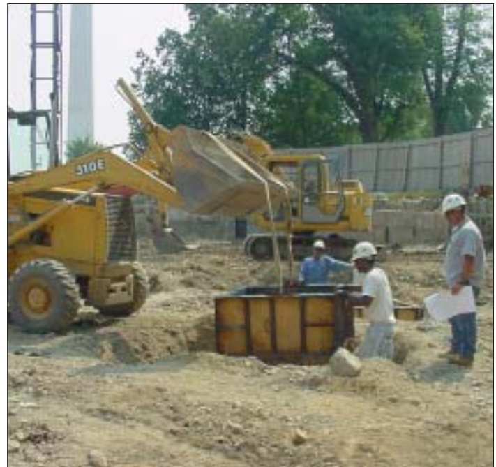
A concrete cap is poured on top of each pile as part of the foundation support structure. (Photo by Stefano Terricola)
