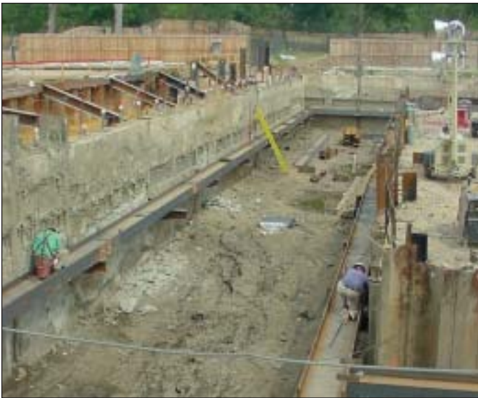
A view of the fountain vault excavation. The vault will house the pumps and valves that control the memorial’s pools and fountains. (Photo by Stefano Terricola)
